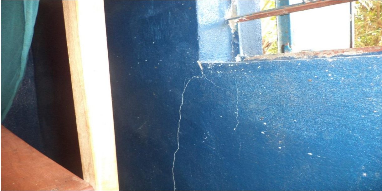
Photo a poorly renovated wall at the Koquima Community Health Post
