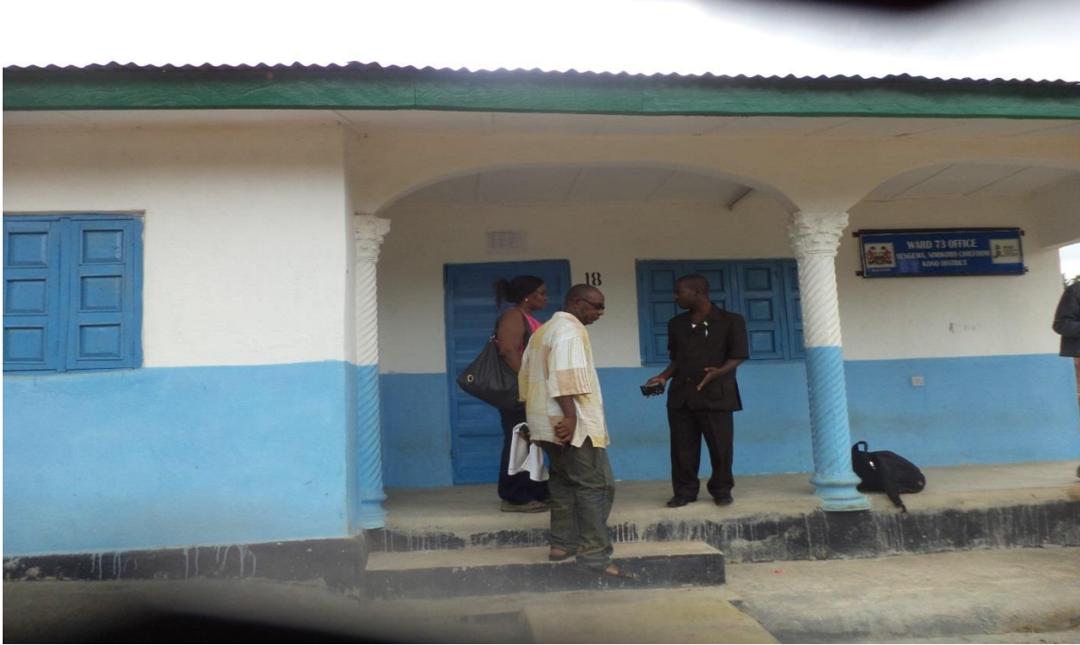
Ward Committee Office constructed by IFAD for Kono District Council with no Notice Board
